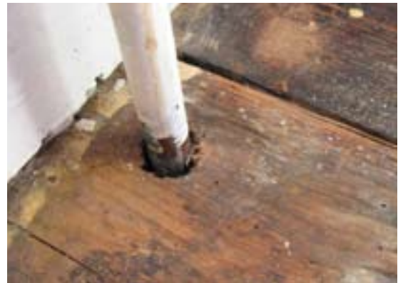
Figure 5 Air leakage through gaps around service pipes in suspended timber floors
