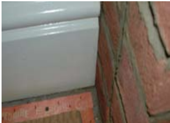
Figure 3 Air leakage path hidden behind skirting board
