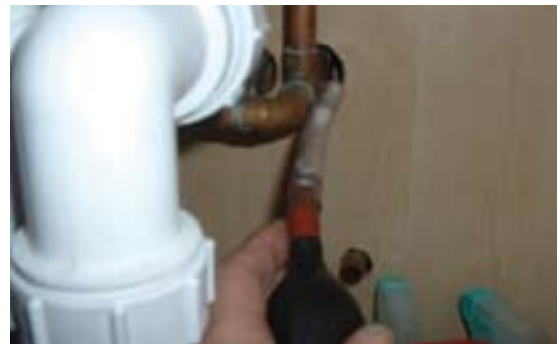
Figure 13 Air leakage around pipes that penetrate the air barrier
