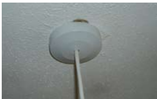
Figure 10 Air can leak through gaps around light fittings into the roof void
