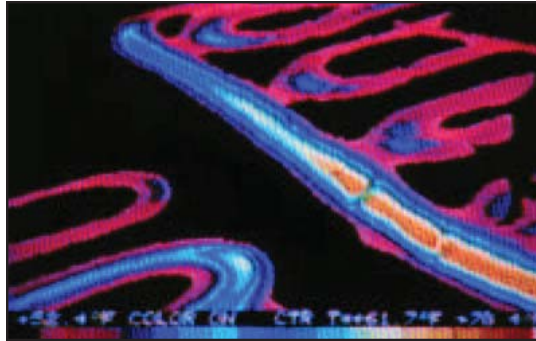
Image 8: Hydronic heating coils embedded in a concrete floor show up in this thermal image.
