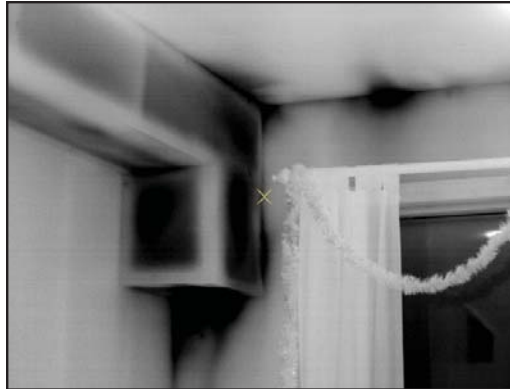
Image 3: The improperly installed fiberglass yields an irregular thermal pattern. The resulting cold spots commonly host wall stains or mold growth.
