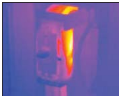
Figure 4: Line-side and load-side lugs are the most common source of abnormal heating, but many breakers have a second set of bolted connections on the back of the breaker. Heat from this connection can be misdiagnosed as the main lug.
